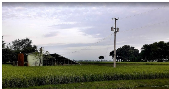
Figure 4: First SIP grid integration piloting site in Bangladesh
